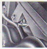
Cooling water drain cock
